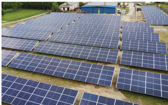
Óhíd (Own power plant) 500 kWp
